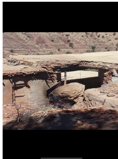
House hit by a falling rock
